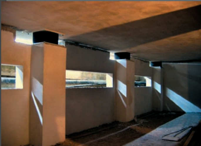
• FOLIGNO, ITALY - Civil Protection Center: installation
